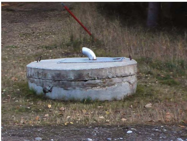
Photo 30 – Sewage lift station at the existing recreation centre site.
