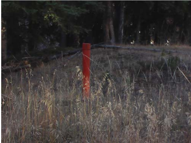
Photo 27 – Monitoring well on CP Rail site at the existing recreation centre site.
