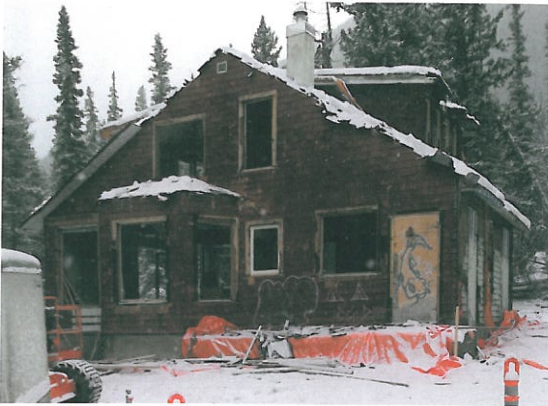
The historic A.O. Wheeler home in Banff on Sunday, Jan. 16, the last day of its existence. Photograph by: Courtesy, Parks Canada
