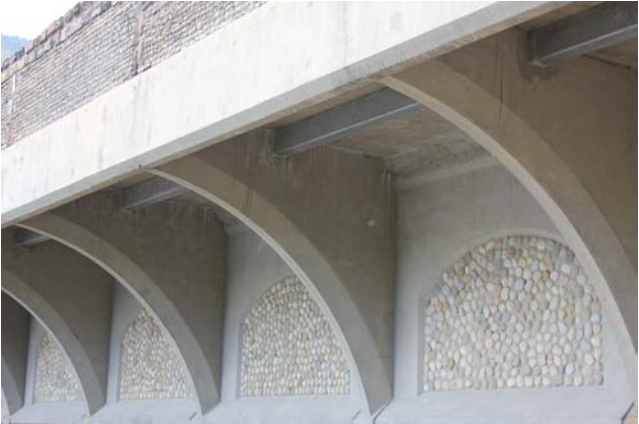
Two Cantilevered Sidewalks
