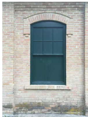
Five (5) 'six over one' Double Hung Round Segmented Windows with Projected Brick Sill and Arched Label Trim.
