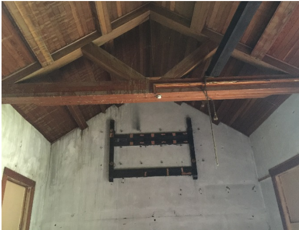
Two (2) Open Web Wooden Trusses in front of Wooden Bracket Supporting Eighteen (18) Insulators
