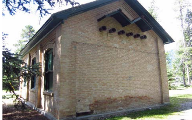
Six Cylindrical Entry Ports under two (2) Arched Covers
